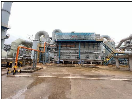
RTO 焚烧系统-焚烧+急冷+碱洗除雾
